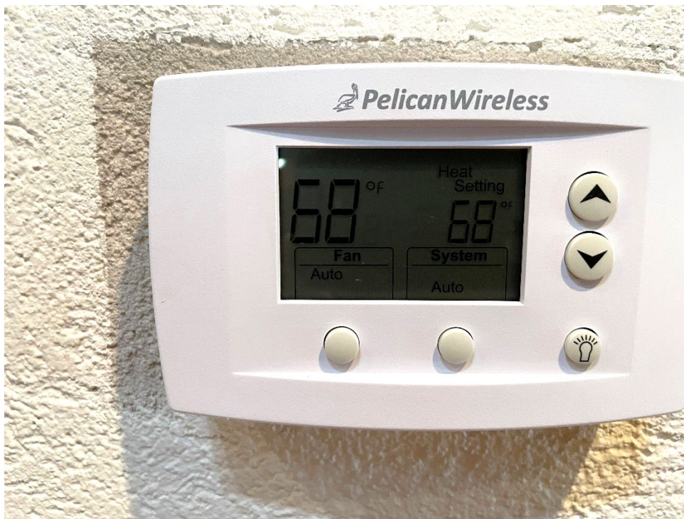
Figure 4 – Existing Standard Programmable Thermostats
